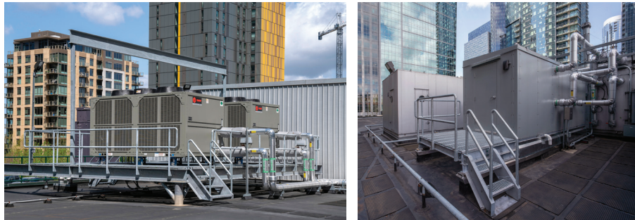
Left: New platform and chillers; Right: New pumphouse
