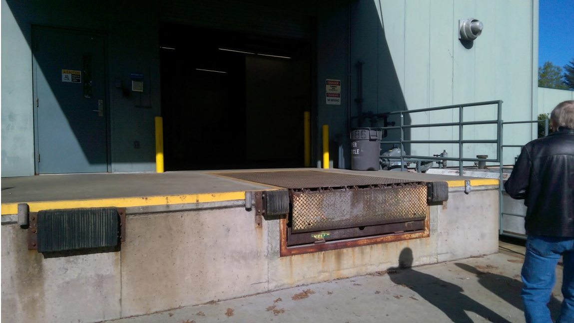
Dock Leveler #4 PHOTOGRAPH 19
