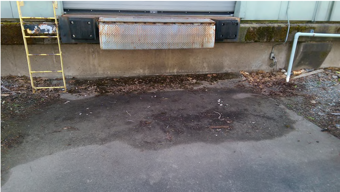
Ponding at Building Wall PHOTOGRAPH 26
