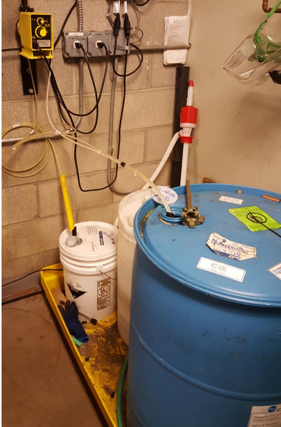
Cooling Tower Treatment System PHOTOGRAPH 05
