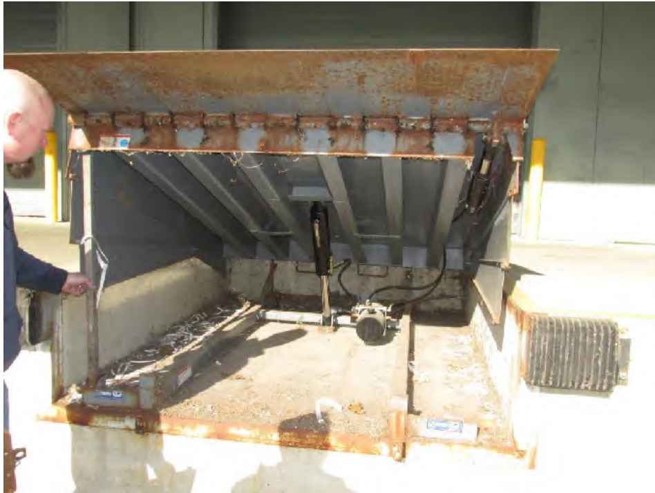
Load Dock Leveler PHOTOGRAPH_03
