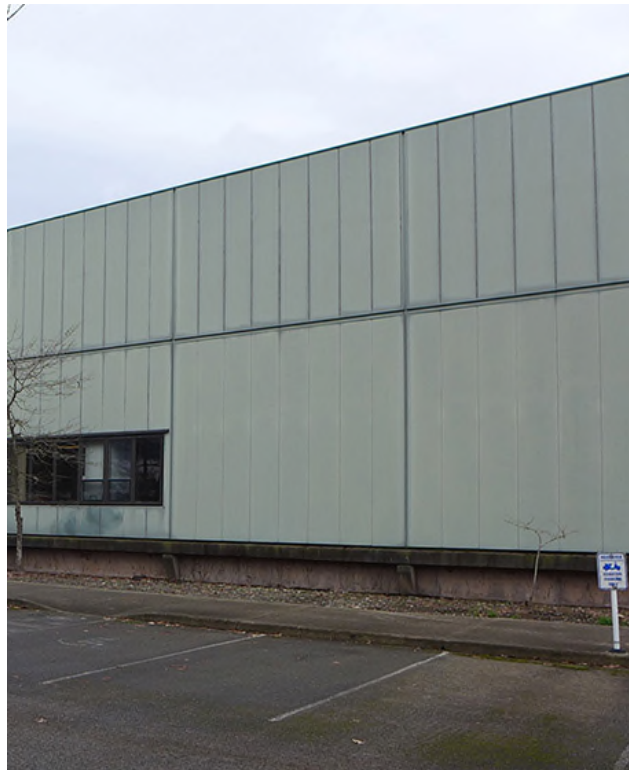
Insulated Panels at High Bay PHOTOGRAPH 14
