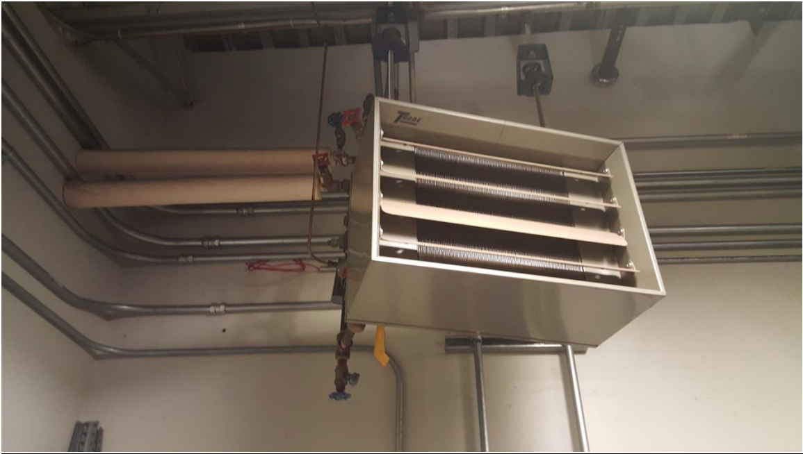
Horizontal Unit Heater PHOTOGRAPH 17
