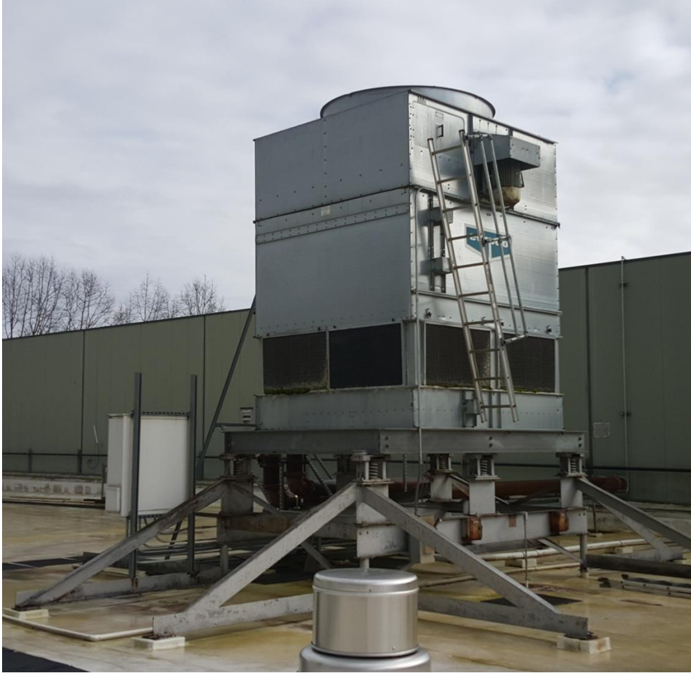
Cooling Tower PHOTOGRAPH 04
