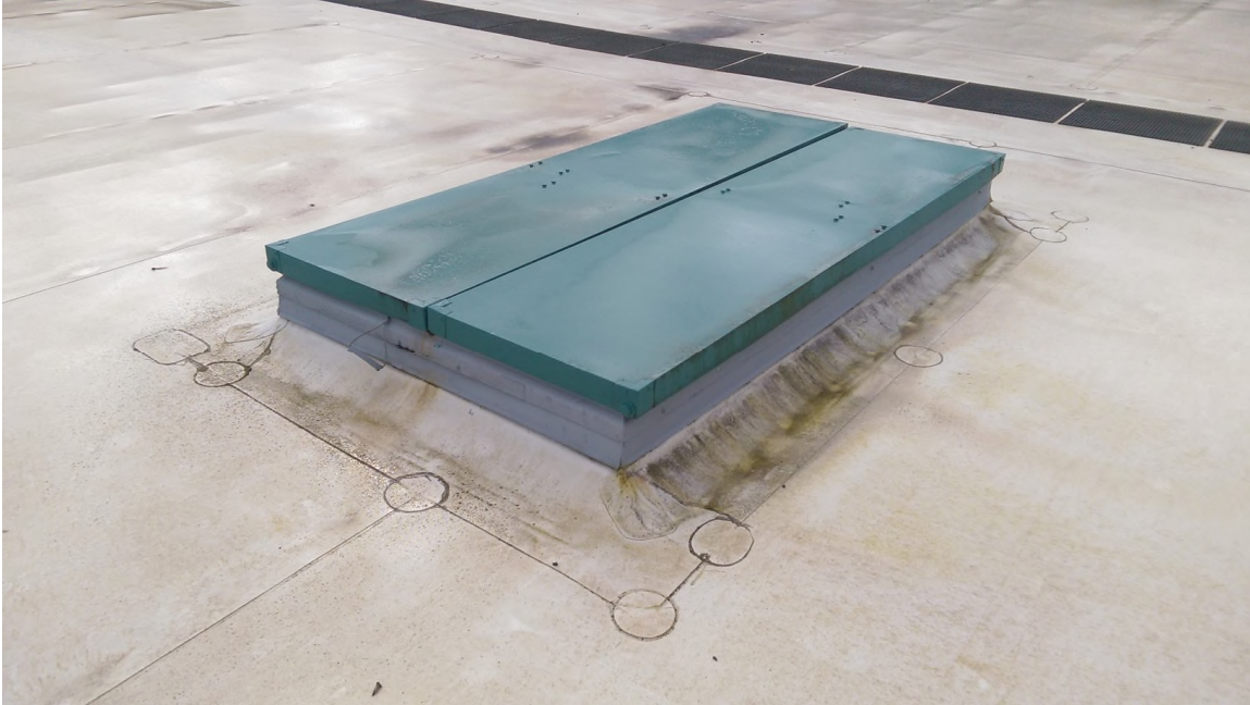
High Bay Ventilator PHOTOGRAPH 9
