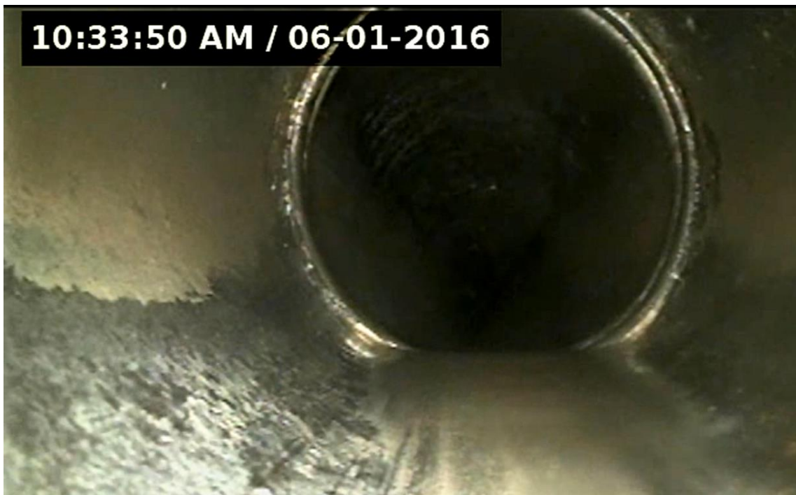
Sewer Lateral Line, PVC PHOTOGRAPH 11
