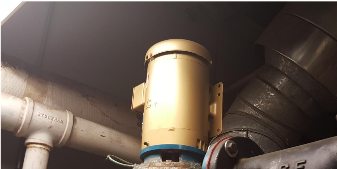
Heating Water Circulation Pump PHOTOGRAPH 07
