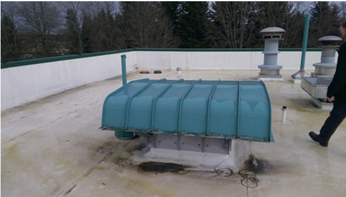
High Bay Exhaust Fan PHOTOGRAPH 10
