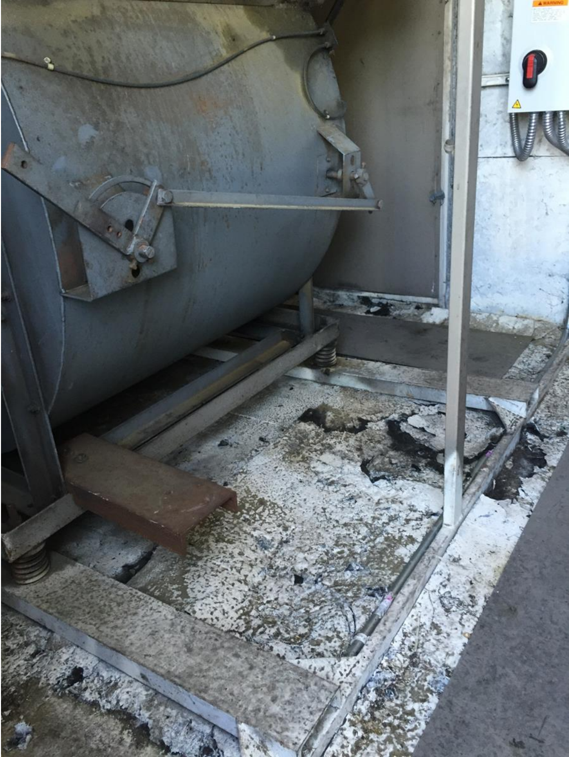
AHU Moisture Damage PHOTOGRAPH 20
