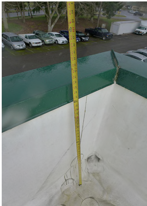
Unsafe Parapet Height PHOTOGRAPH 12
