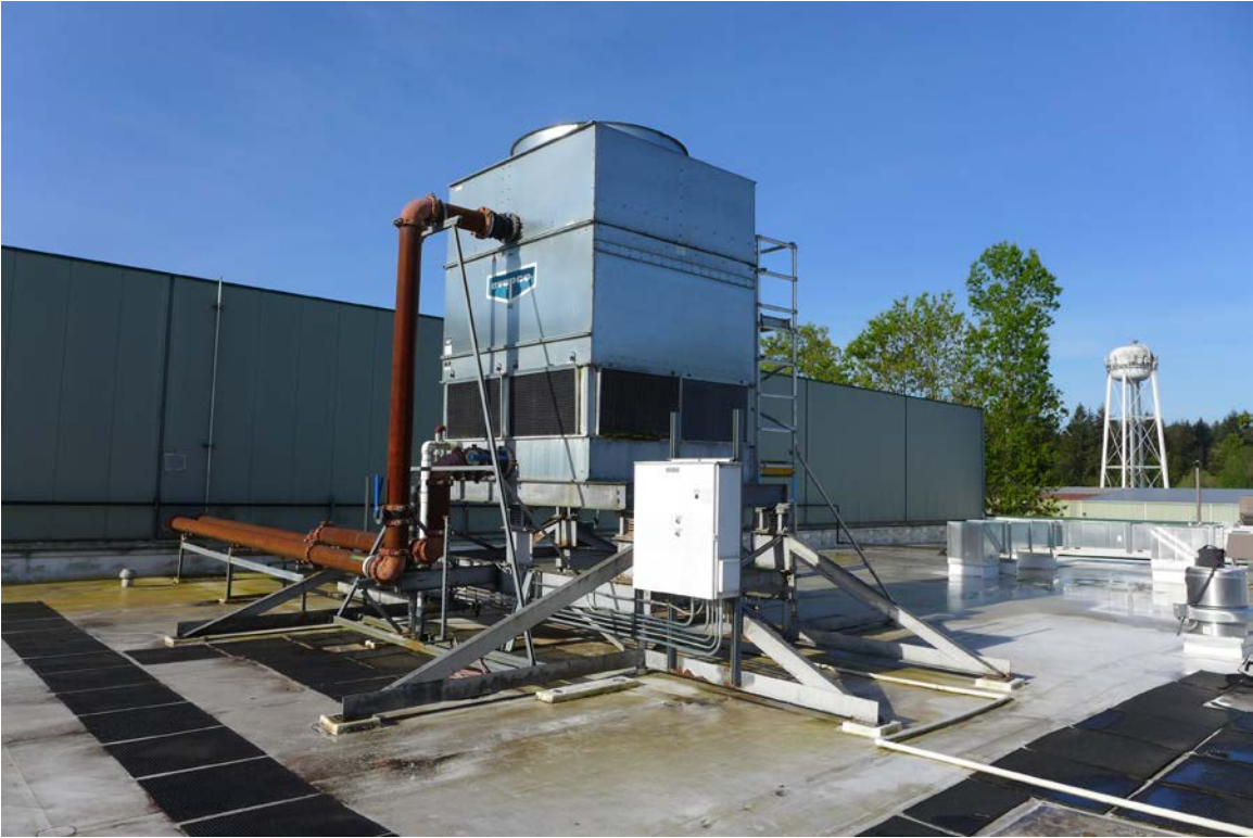
Cooling Tower PHOTOGRAPH 5
