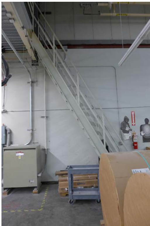
Mezzanine Ships Ladder PHOTOGRAPH 11
