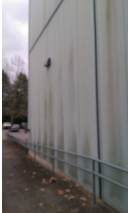
Insulated Panel Mold Growth and Discoloration PHOTOGRAPH 15
