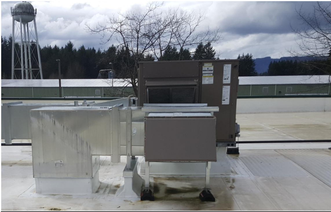
New Air Handling Unit PHOTOGRAPH 02
