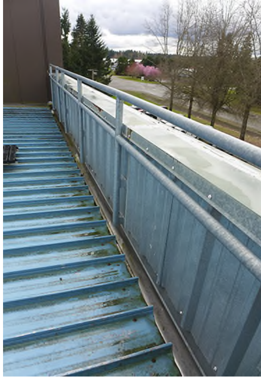
Fall-Protection Guardrail at Adjacent Isabella Bush Building PHOTOGRAPH 13
