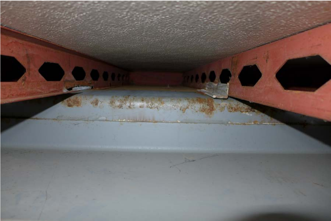
Parapet Cavity PHOTOGRAPH 4
