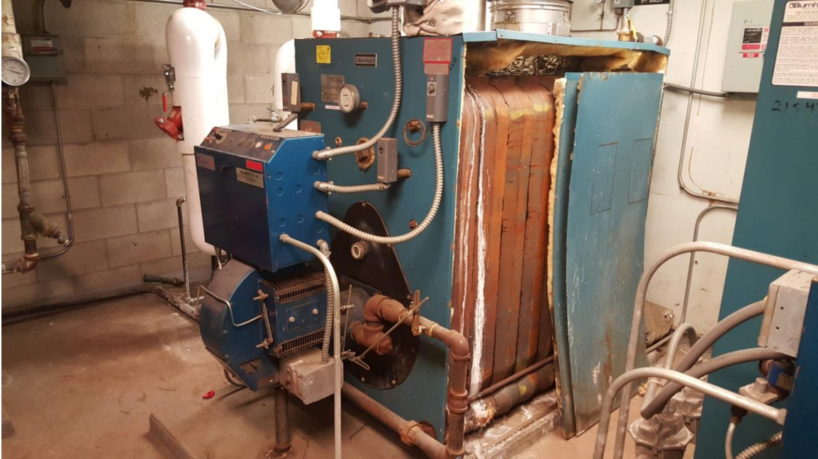
Heating Water Boiler PHOTOGRAPH 06
