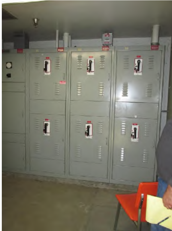
Elect Rm 704 - Main Switchboard 2500Amps PHOTOGRAPH 01
