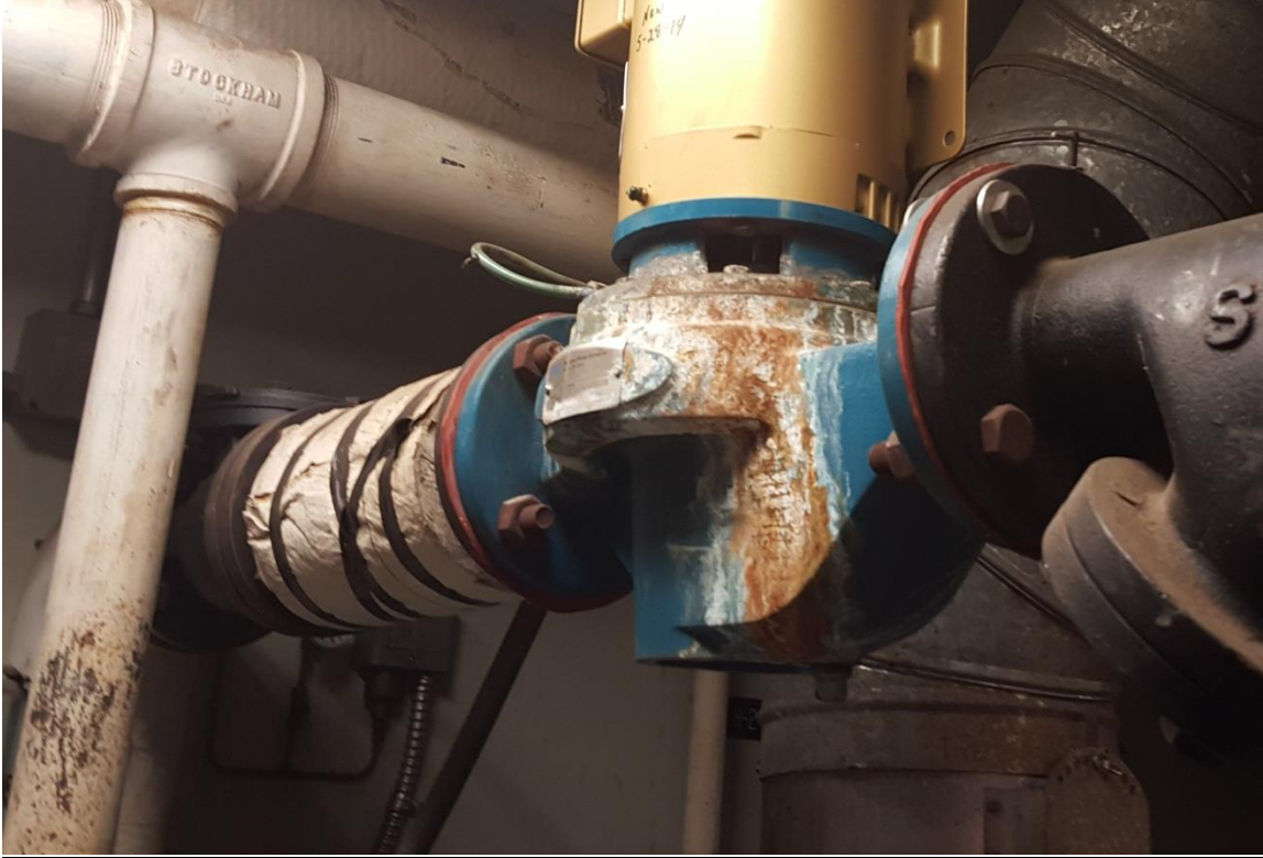
Signs of Rust and Scale in Pipes PHOTOGRAPH 21
