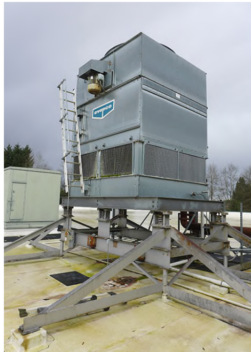
Low Bay Cooling Tower PHOTOGRAPH 6
