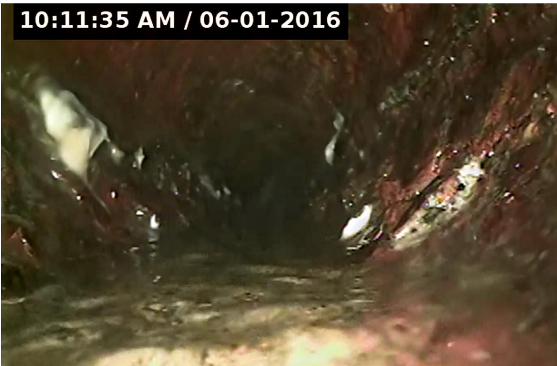
Waste Line, Cast Iron PHOTOGRAPH 13
