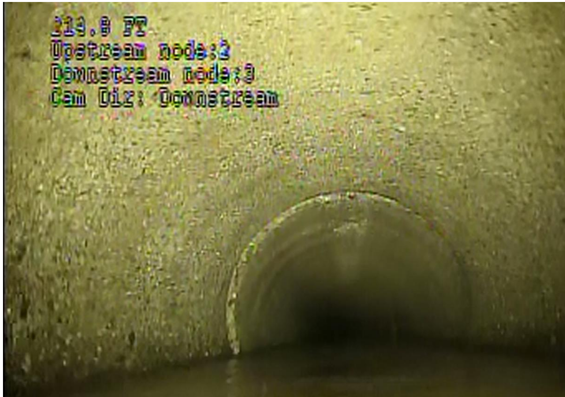
Sewer Main Line, Cement PHOTOGRAPH 10
