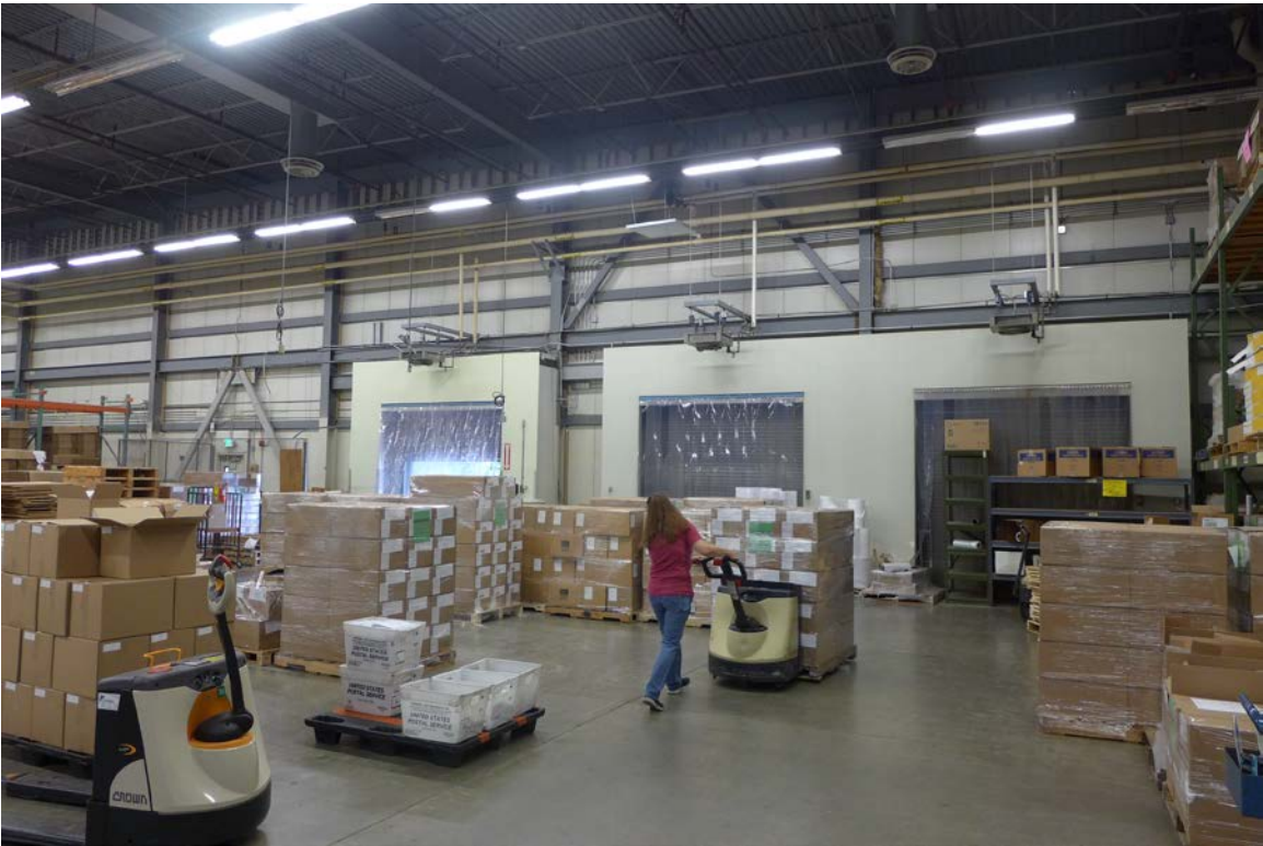
Offset Braces Resulting in Vertical Irregularity PHOTOGRAPH 16
