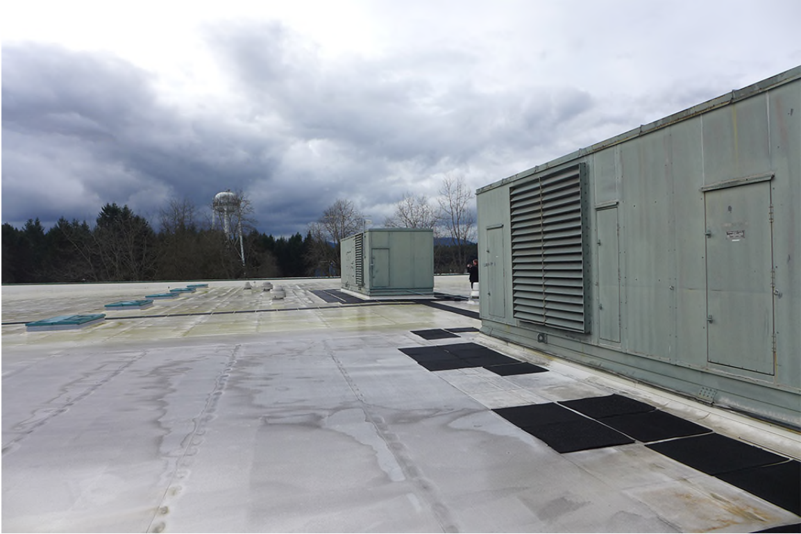
High Bay HVAC Equipment PHOTOGRAPH 7
