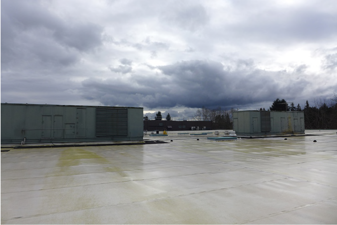
Low Bay HVAC Equipment PHOTOGRAPH 5
