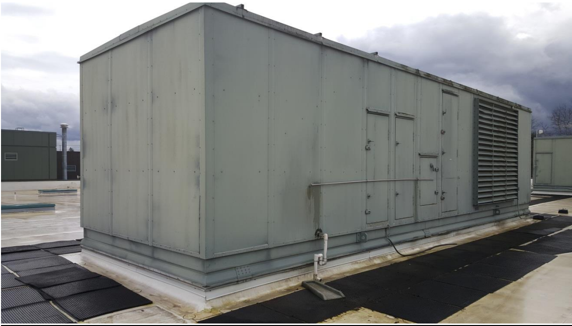
Typical Air Handling Unit PHOTOGRAPH 01
