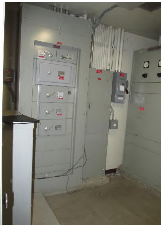
Elect Rm 704 - Switchboard 'HA' 800Amps PHOTOGRAPH 02
