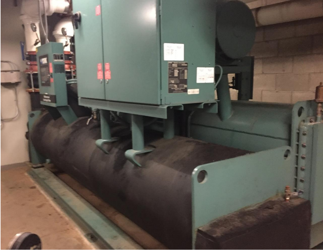
Centrifugal Chiller PHOTOGRAPH_03
