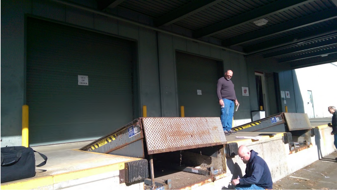
Dock Leveler #2 PHOTOGRAPH 17
