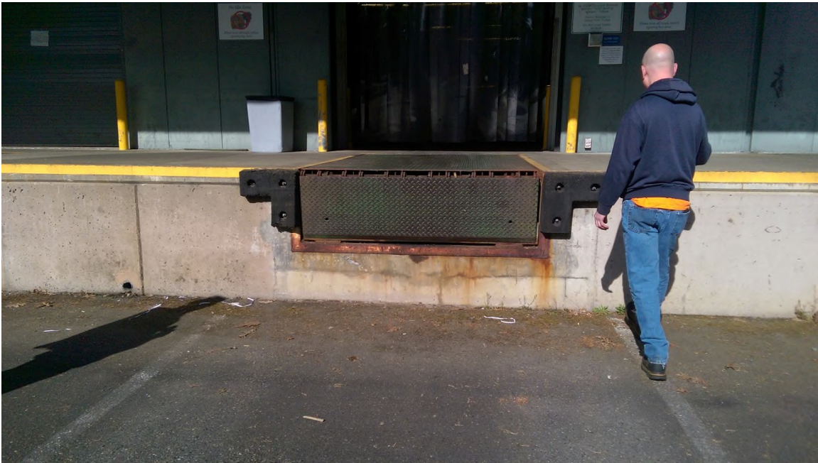
Dock Leveler #3 PHOTOGRAPH 18
