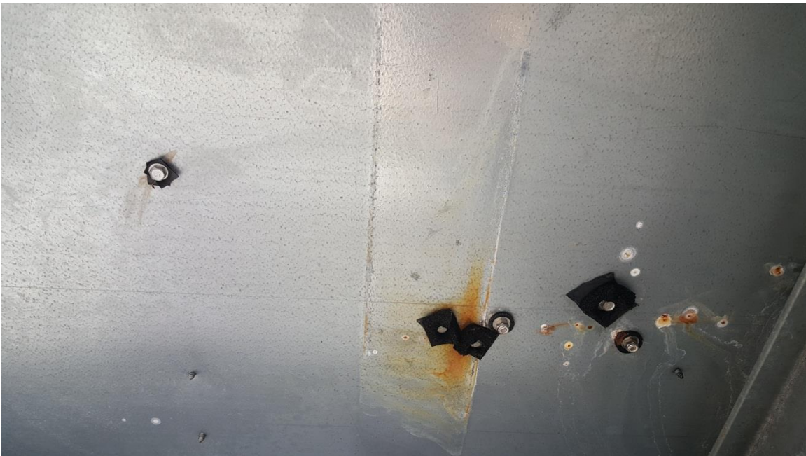
Cooling Tower Leak Damage and Patches (View of Bottom of Tank) PHOTOGRAPH 22
