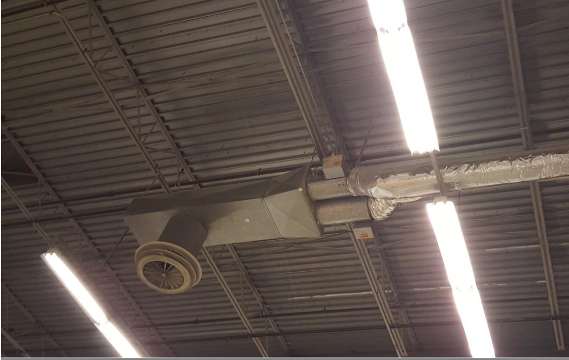
Air Terminal Unit PHOTOGRAPH 16
