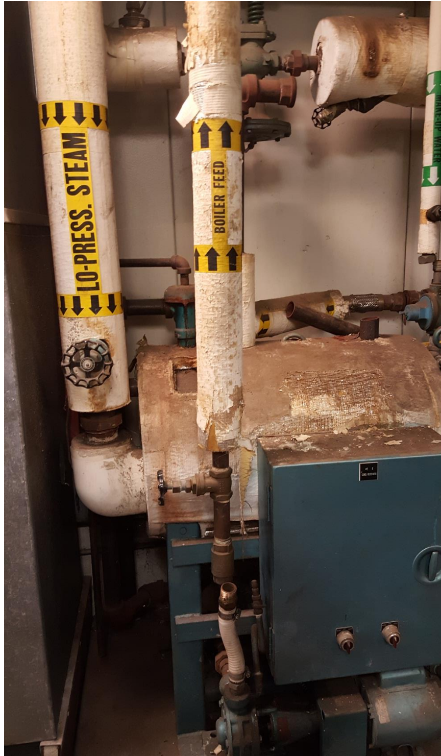
Abandoned Steam Condensate System PHOTOGRAPH 15
