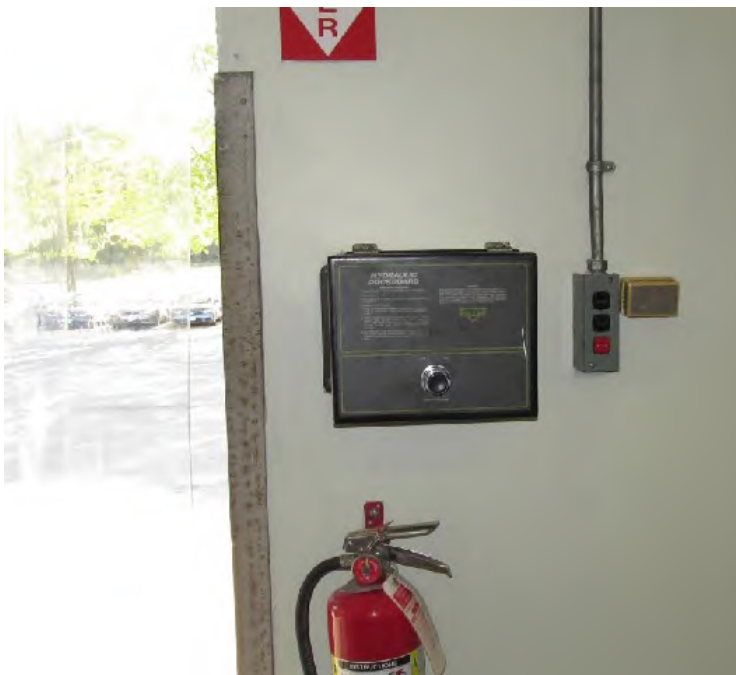
Load Dock Leveler Controller PHOTOGRAPH_04
