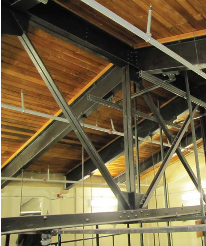
Figure 50: Steel and utilities in Skylight Attic
