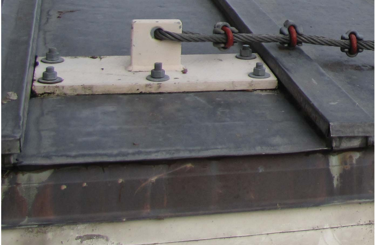
Figure 59: Detail of roof tie-off system and staining of perimeter copper flashing
