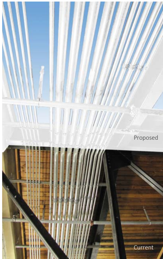
Figure ES06: Photo showing proposed reflective white paint on all surfaces of the skylight attic with glazing above
