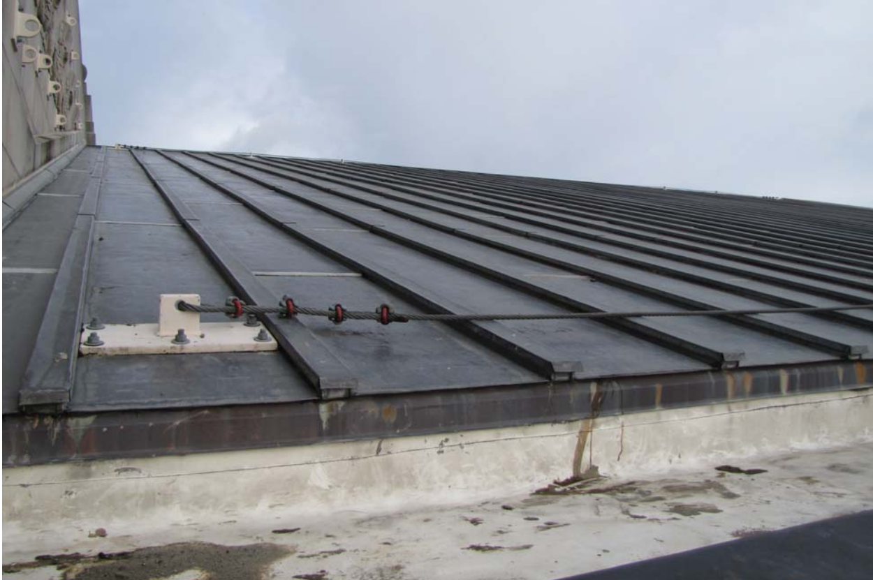
Figure 29: Existing batten seam roof. Corrosion is visible at the perimeter flashing.
