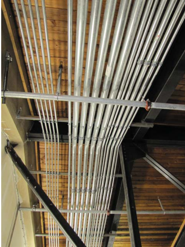
Figure 27: Conduit and piping runs along one of the bays
