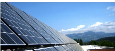
Angst Hall, Skagit Valley College. Sustainable features support active use, manage rainwater, collect natural power, and engage the outdoors.
