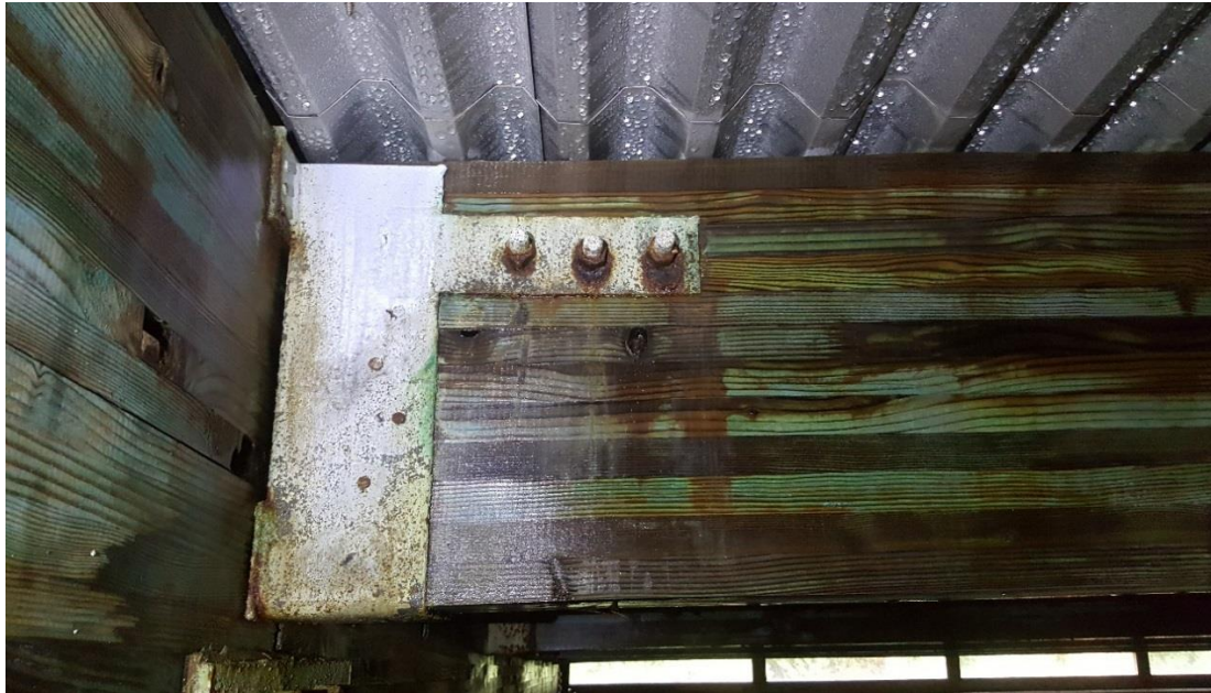
Typical Corroded Purlin Hanger
