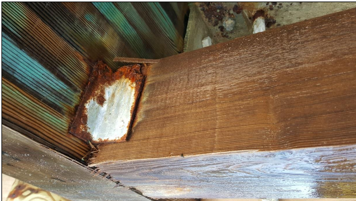
Typical Corroded Hanger and Fasteners at Blocking
