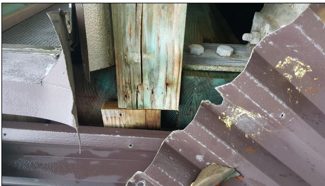
Corroded Metal Decking Panels at Fastener Attachment Points
