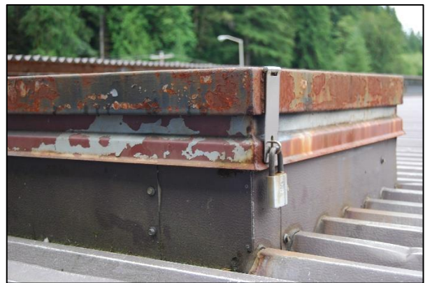
Rust at Access Hatch in Northwest Corner
