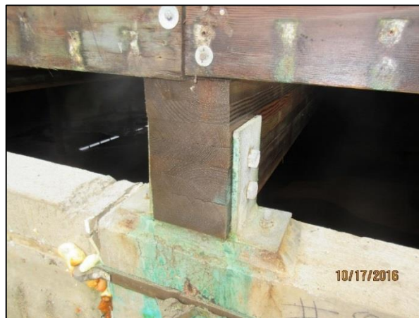
Typical Delamination of Glulam Purlins
