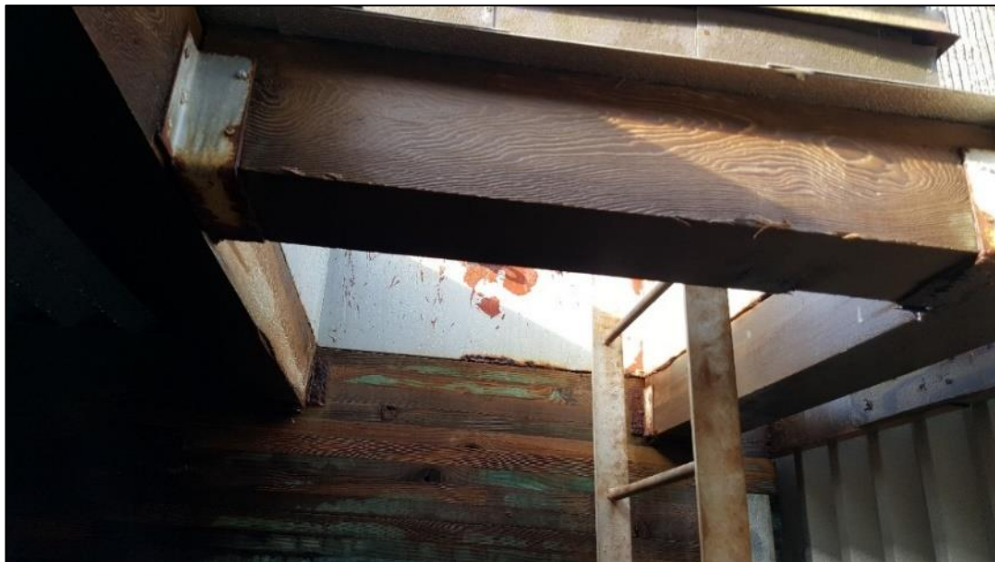
Corroded Hangers at Access Hatch Blocking
