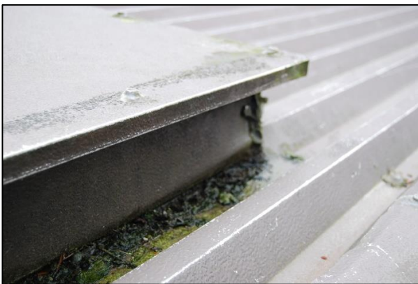
Mold/Mildew at Equipment Hatch Flashing
