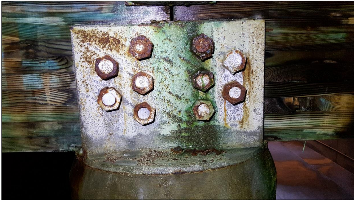
Typical Corroded Hanger and Fasteners at Girder Support Column
