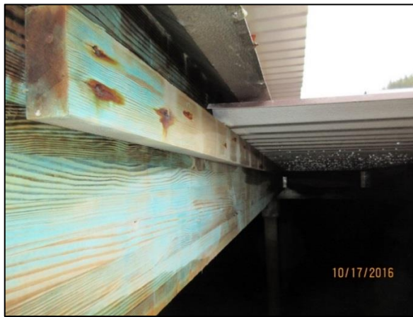
Detached 2x4 Decking Support Ledger at Rim
