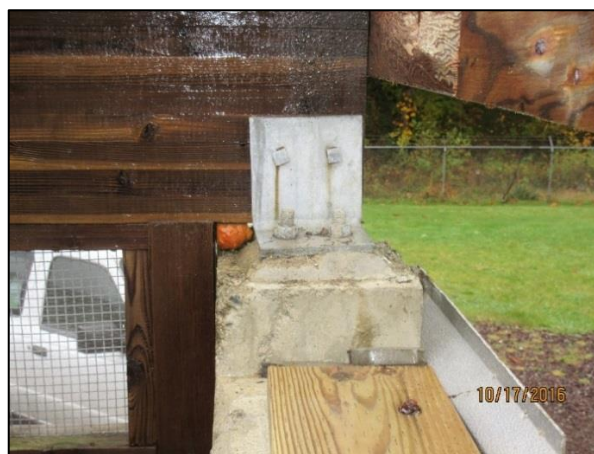
Signs of Corrosion in Perimeter Glulam Beam
