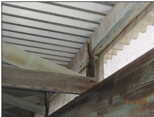
Typical Corroded Hanger and Fasteners at Pop-up Ridge Structure
