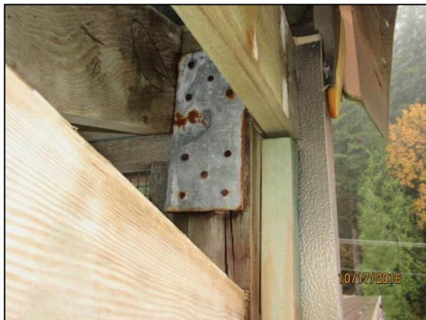
Typical Corroded Hanger and Fasteners at Ridge
