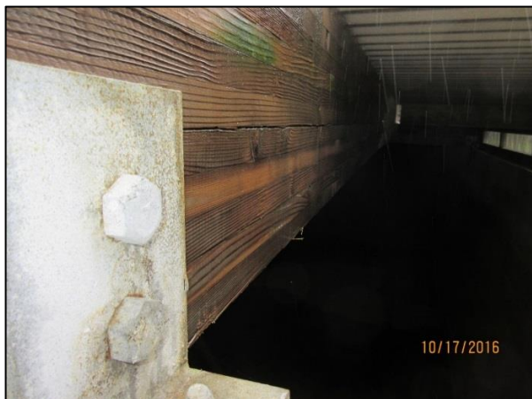
Typical Delamination of Glulam Purlins
