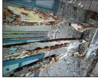
Residential High-Rise Envelope Failure – Steel Stud Corrosion
