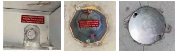
REFERENCE IMAGES: SEALED PENETRATIONS TO ASBESTOS CONTAMINATED CONDUIT (NOT SHOWN, EXISTS THROUGHOUT FLOORS 1, 2, & 3)
