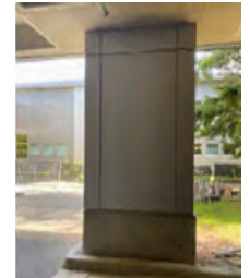
P1: ASBESTOS CONTAMINATED EXTERIOR COLUMN CAVITY
