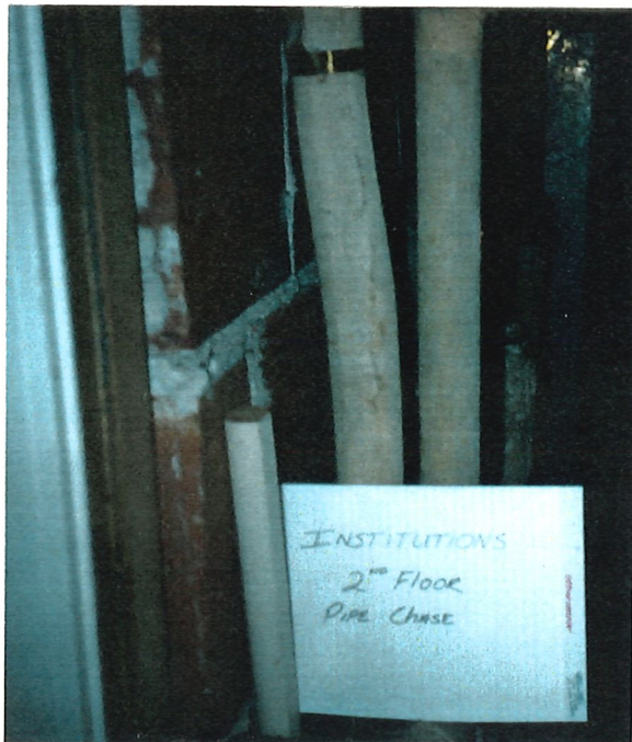
ASBESTOS-CONTAINING FELT WRAP PIPE INSULATION; SECOND FLOOR PIPE CHASE AT ATTIC ACCESS.
