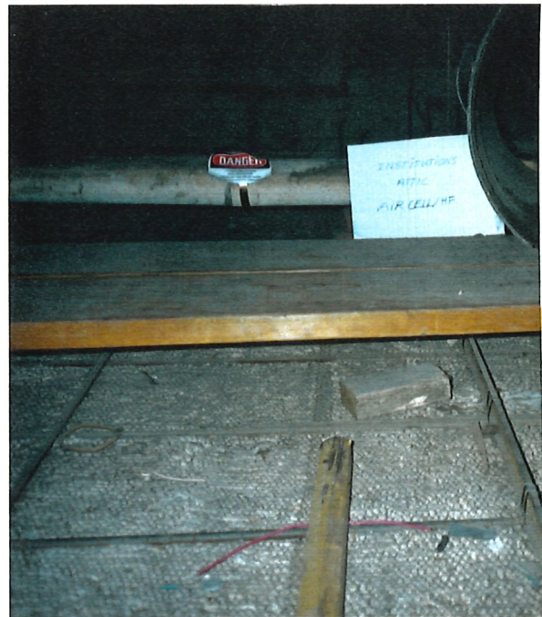
ASBESTOS-CONTAINING AIR CELL PIPE INSULATION; ATTIC CRAWLSPACE AT ROOF ACCESS.
