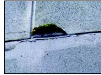
Fig. 3.1.4 2002 photograph of plant growth along the joints on the west facade of the stacks. Photograph by Artifacts Consulting, Inc.
