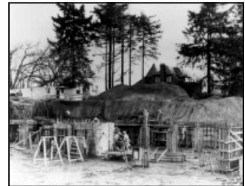
Fig. 1.2.7 Ca 1957 photograph of the Library construction, looking southeast at the excavated site. Photograph courtesy of the Washington State Archives.
