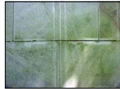
Fig. 3.1.5 2002 photograph of repairs on the west facade of the stacks. Photograph by Artifacts Consulting, Inc.
